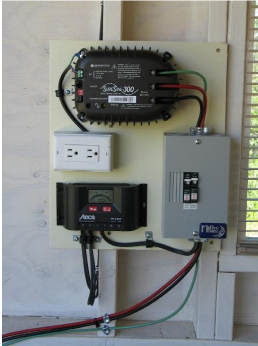
Figure 6. Solar power control system.
